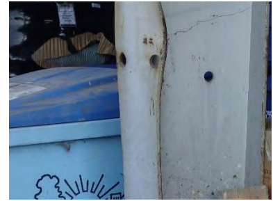
Figure 11: Storage Shed, Warped Column Flange
