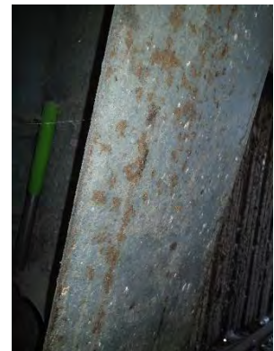
Figure 31: MRF, Rusted Steel Column
