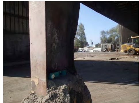
Figure 3: TS East Wall, Warped Column Flange
