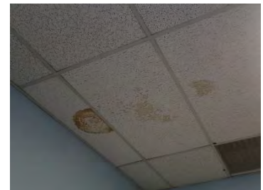
Figure 18: Admin Office, Water Stain on Ceiling Tiles
