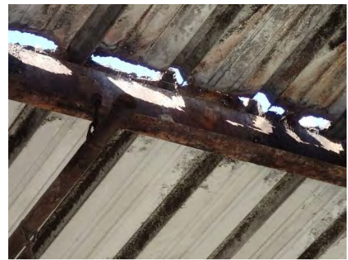
Figure 6: TS Corroded Roof Deck & Roof Purlins
