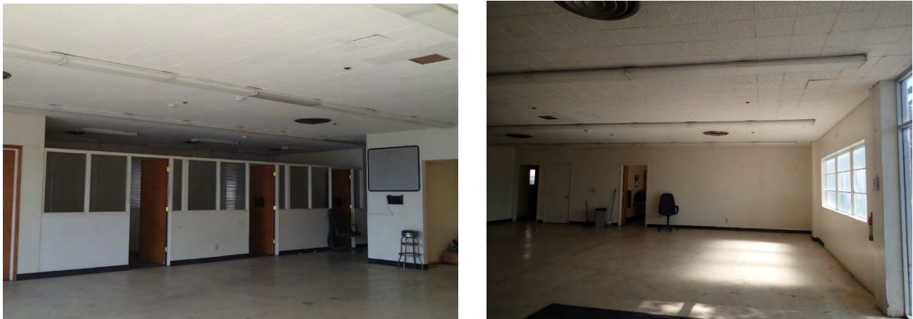
Figure 21 & 22: Concrete Building, Offices, Interior View (Left) & Concrete Building, Offices, Interior View (Right)
